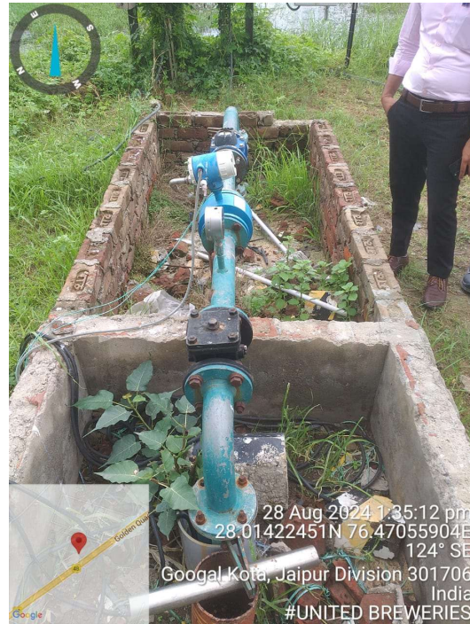
Figure 7 : Photograph of Bore Well.
