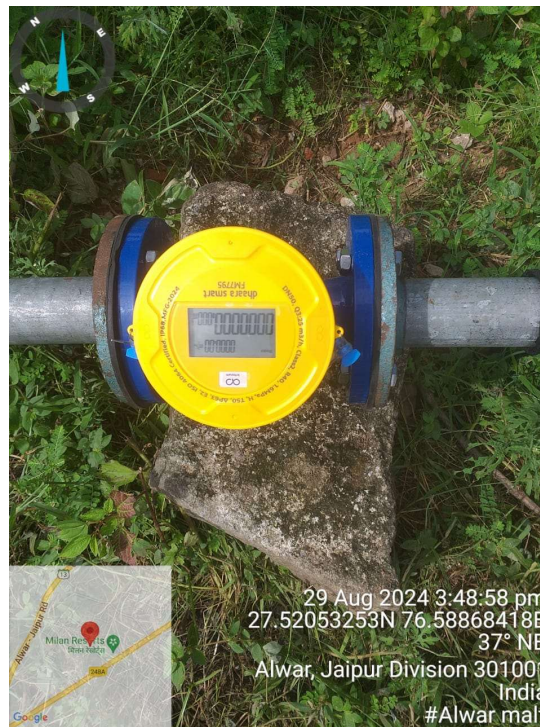
Figure 13: Photograph of flowmeter.
