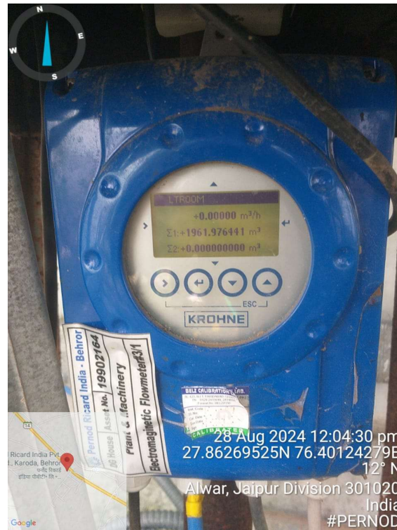
Figure 5 : Photograph of Bore Well flowmeter with telemetry.
