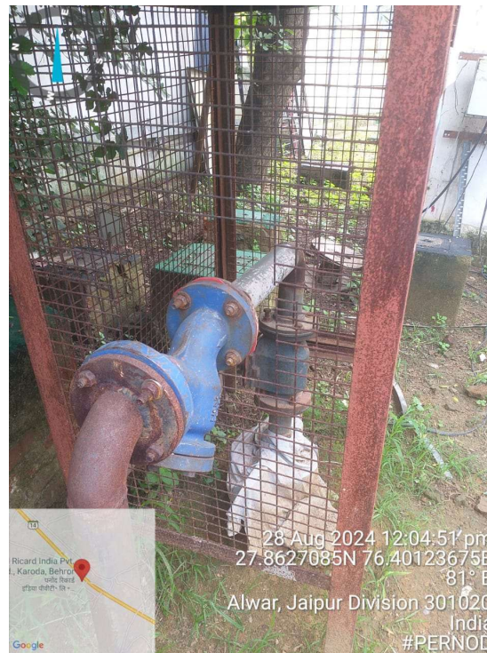
Figure 6 : Photograph of Bore Well.
