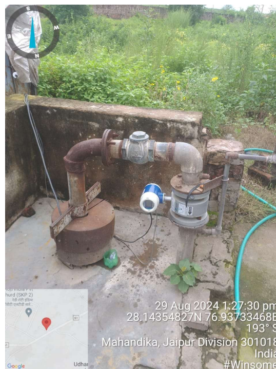
Figure 12: Photograph of Bore Well with flowmeter.
